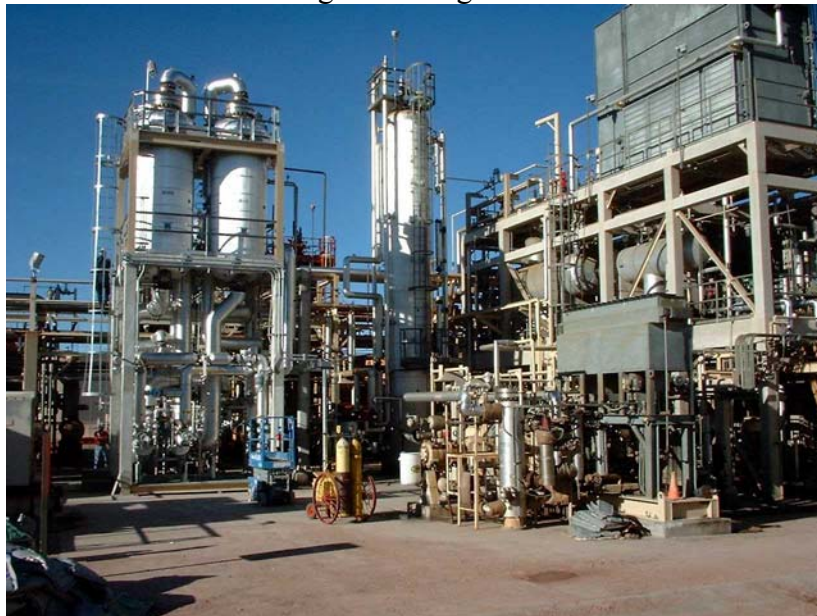
Figure 6 A View of the IsoTherming Unit Integrated into the Ciniza Refinery
